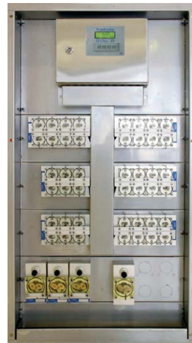
Panel with OVAL D, SR blocks, and SR single meters, (see pages 11–12).
